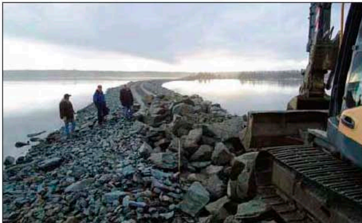
A major reconstruction project on the Salt Marsh Trail is currently ongoing. (SUBMITTED)
